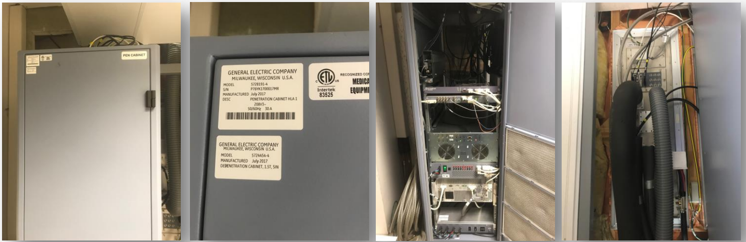
PEN Cabinet HLA1 & Penetration Panel – P/N: 5728191-4 S/N: P76YK1700017MR
